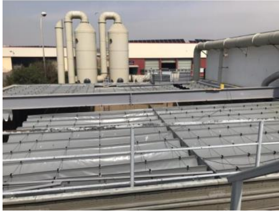
Figure 22: Bassin tampon couvert
