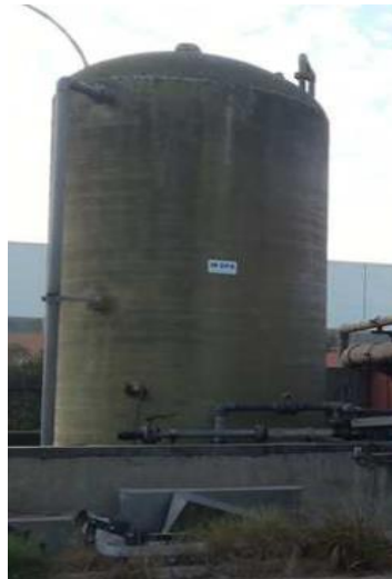
Figure 11: Stockage des graisses existant[7]
