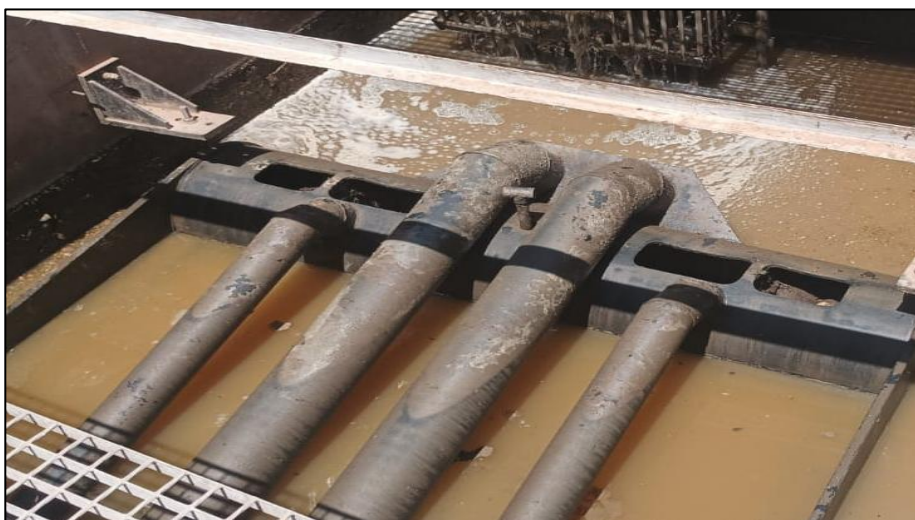
Figure 13 : Siphon mécanique (Asselda)
